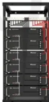
Cabinet and rack installation display
